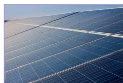
Photovoltaic / semiconductor wafer industries
